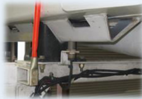
Proximity switches at multiple locations
