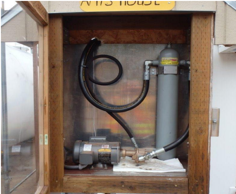
Fuel Polisher Filter and Motor
